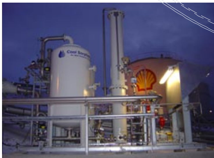
Gasoline Vapour Recovery Unit (VRU) installed at Hammerfest, Norway
