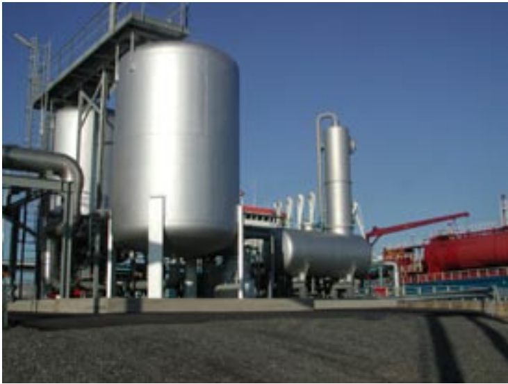
Newly built VRU at Gothenburg, Sweden
